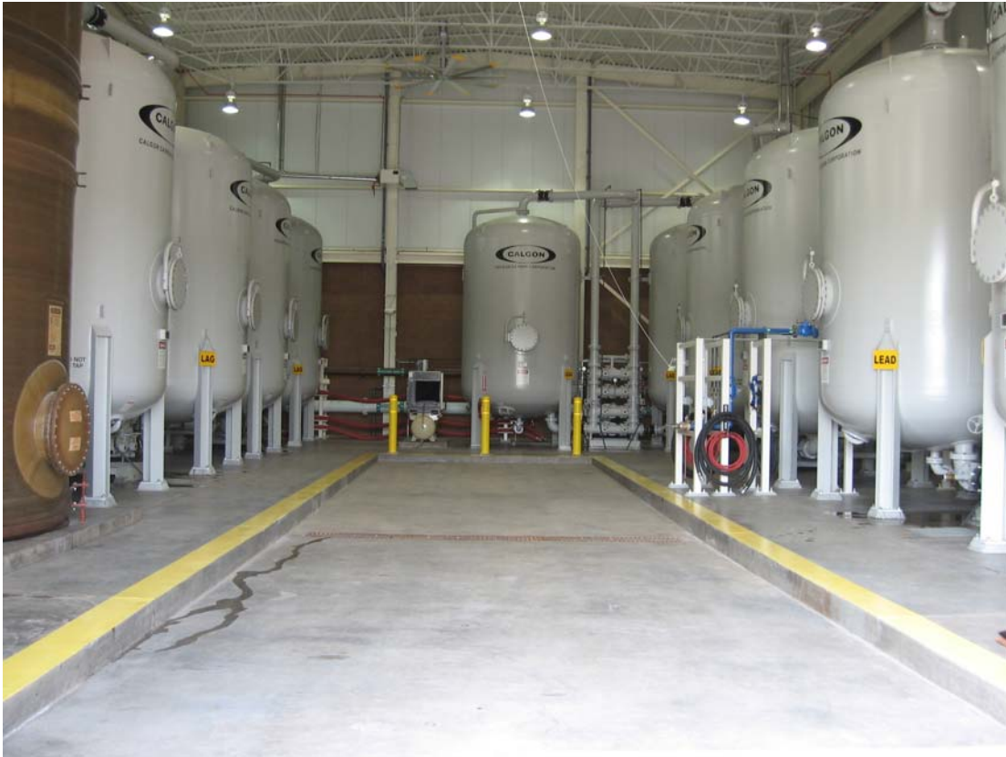
Figure 14: Oakdale Water Treatment Plant
