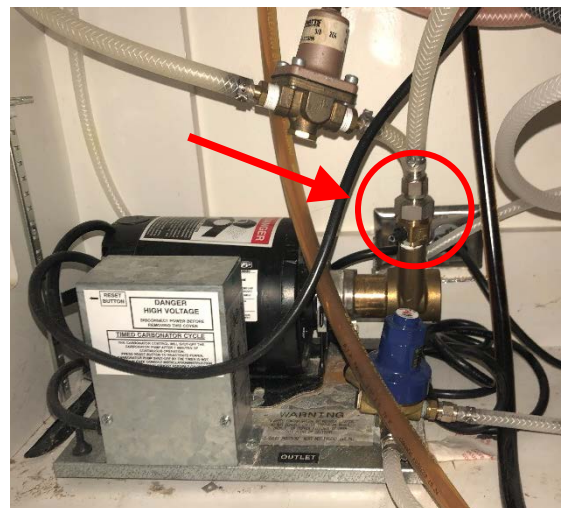
One example of an ASSE Standard 1022 approved backflow prevention device. Devices may vary in appearance. Devices should be labeled ASSE 1022.
