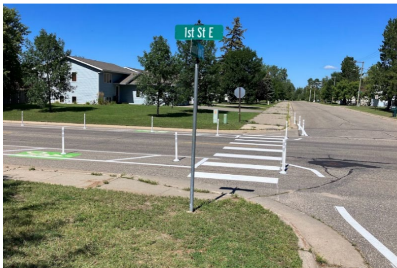
Figure 4: Installed Demonstration Project
